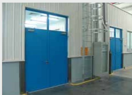
⑧ Fire-rated Doors
